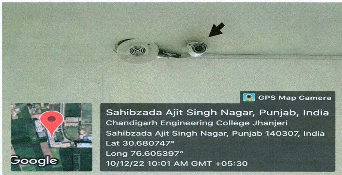
CCTV Camera in Corridor
