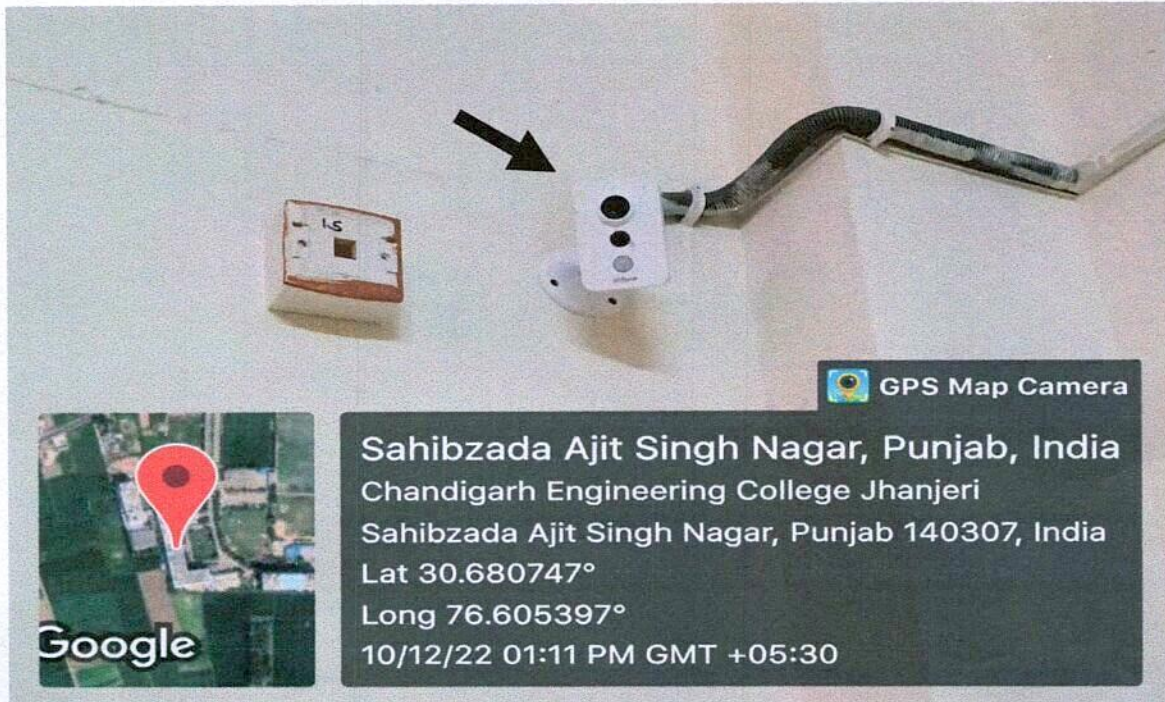
CCTV Camera with Mic in the Classroom
